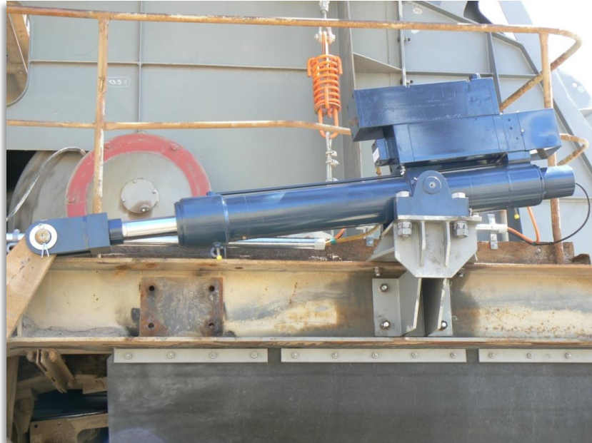
Guidance of the material flow via flap operation
